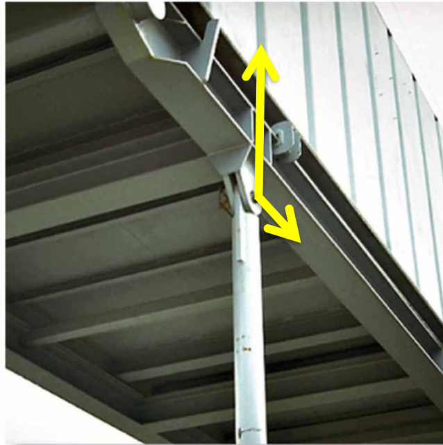
unfig05_04.jpg - This utility building is pin supported at the top of the column. (8) This utility building is pin supported at the top of the column. (8)
